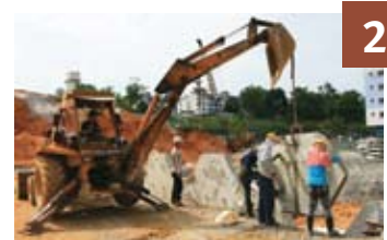
The first course of facing panels are placed on the levelling pad. The hexagonal facing panels are made of precast concrete and interlocked with dowel bars.
