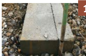
The first step is to remove unsuitable subsoil material and replace it with well-compacted granular material. A concrete levelling pad is installed at the formation level.
